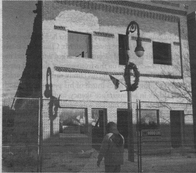
The Dunlay building in downtown Marmora was demolished on December 22 amid the busy Christmas shopping rush. Members of the demolition team made sure no one got too close to the falling debris while the operator manned the demolition equipment. Photo: Cindy Redding
